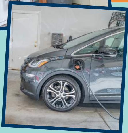
Heat Pump Water Heater & Electric Vehicle Charging
