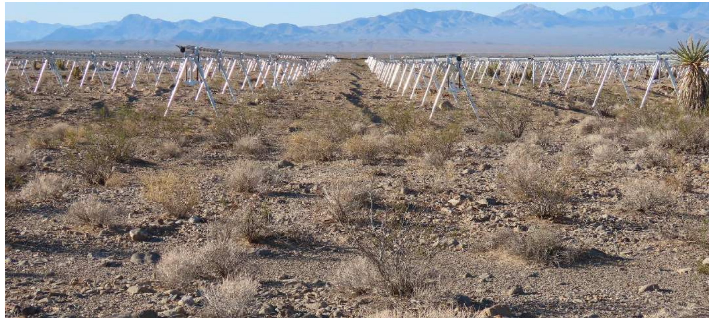
Yellow Pine Solar + Storage 50 MW COD June 2023
