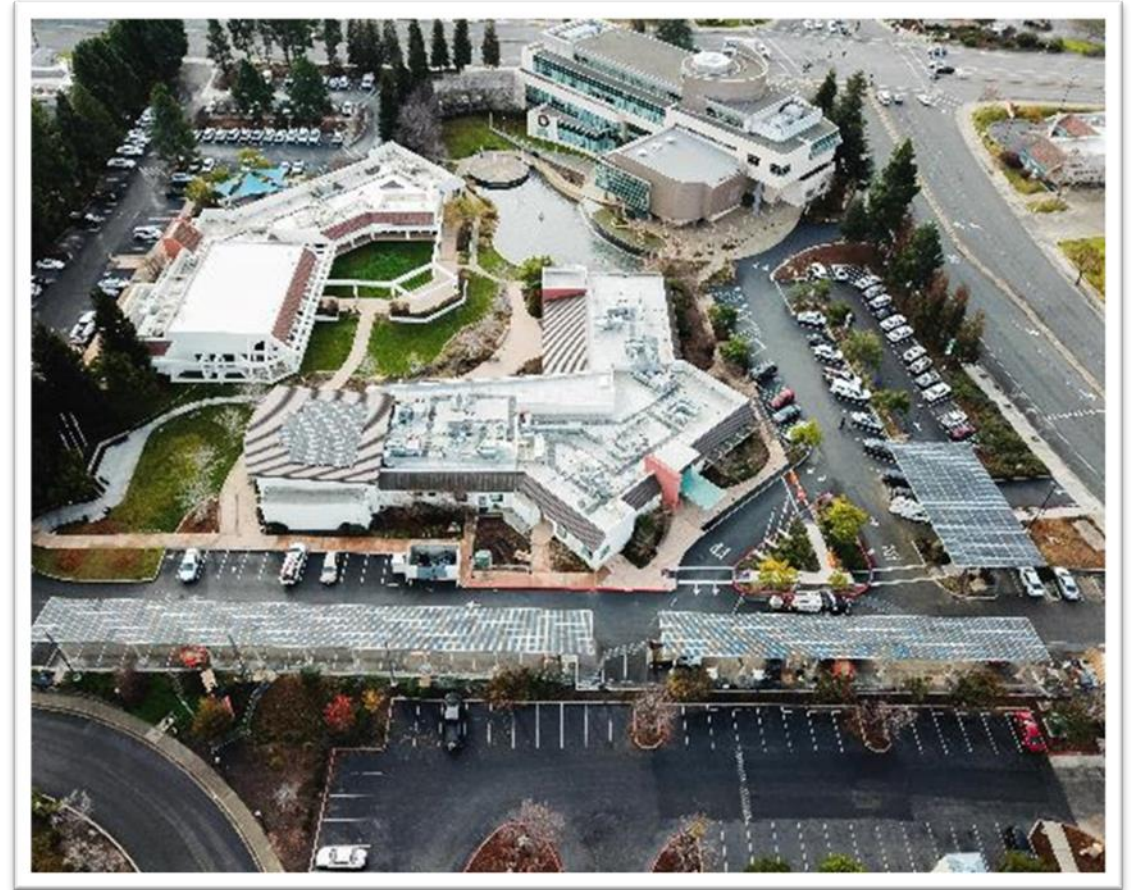
Solar + battery installed at Milpitas' Community & Senior Center
