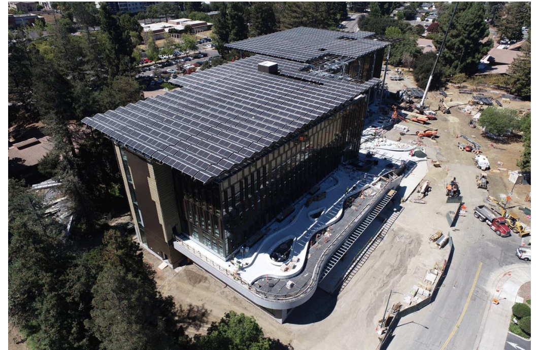
Solar + battery installed at Sunnyvale's City Hall
