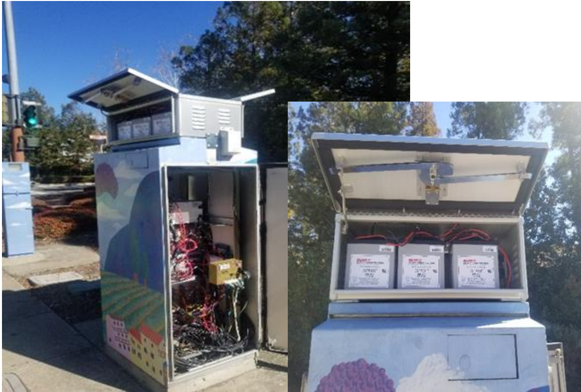
Battery backup at traffic light signals throughout city
