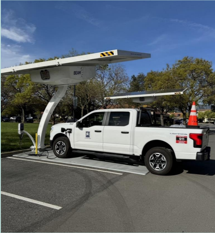
Cupertino used its Community Resilience Grant to purchase off-grid EV chargers
