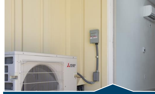
Turnkey Single Family Electrification Service (including emergency water heater)
