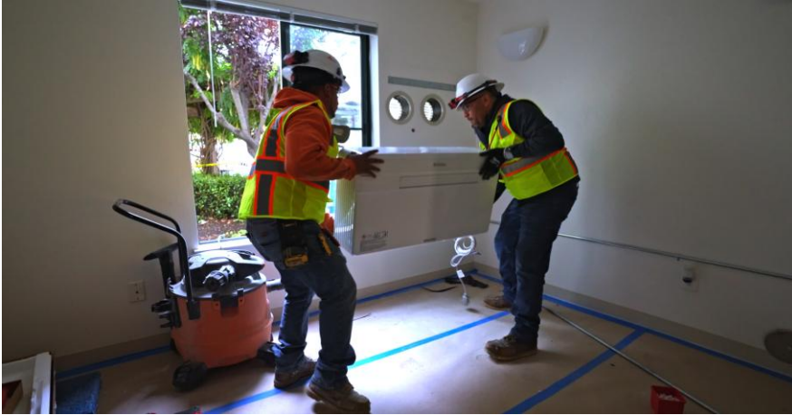
Heat pump installation at Sunnyvale site with no previous AC
