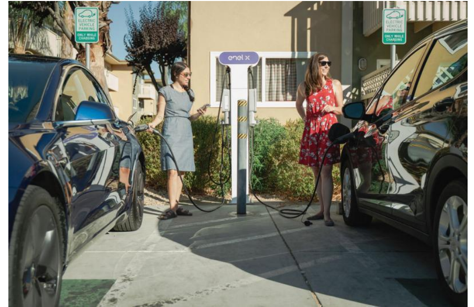
SVCE-funded EV chargers at a multifamily site in Mountain View
