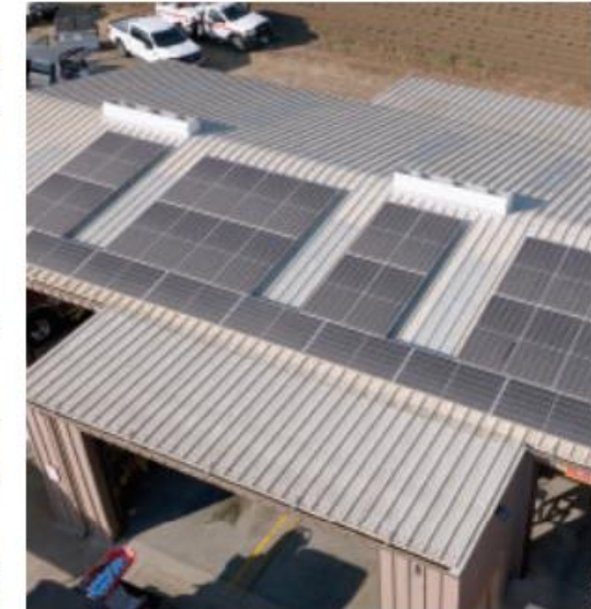
ROOFTOP POWER The new solar energy system at Masten Station, pictured July 10, will equip the facility to operate during power outages and save money for the publicly funded South Santa Clara County Fire District.
