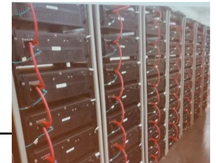
Smart Microgrid + Second life Li-Ion Energy Storage
