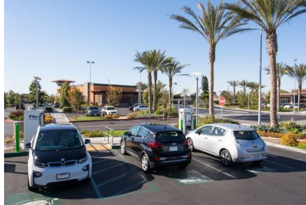
Gen 2 Charging Station 50 kW 2-4 chargers
